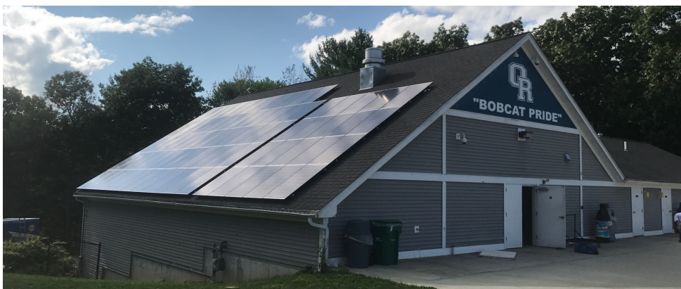
Solar array on service building that was completed in 2017
